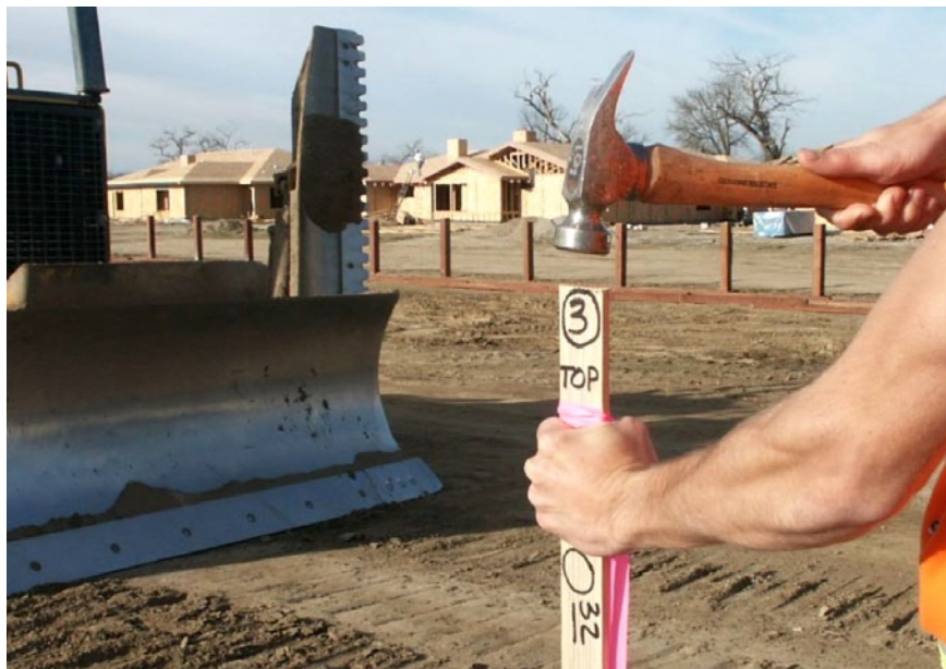
A surveyor hammering in a piece of wood lath on a job site describing offsets, the amount of material to cut or fill and the point identification.
